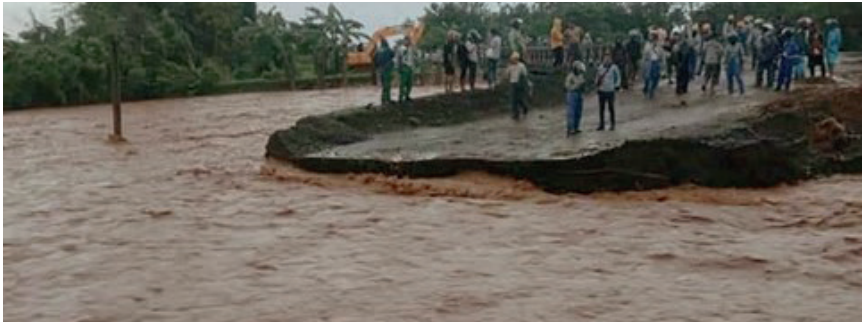
Figure 4.12: Bridges in Bahodopi destroyed by floods in July 2020
